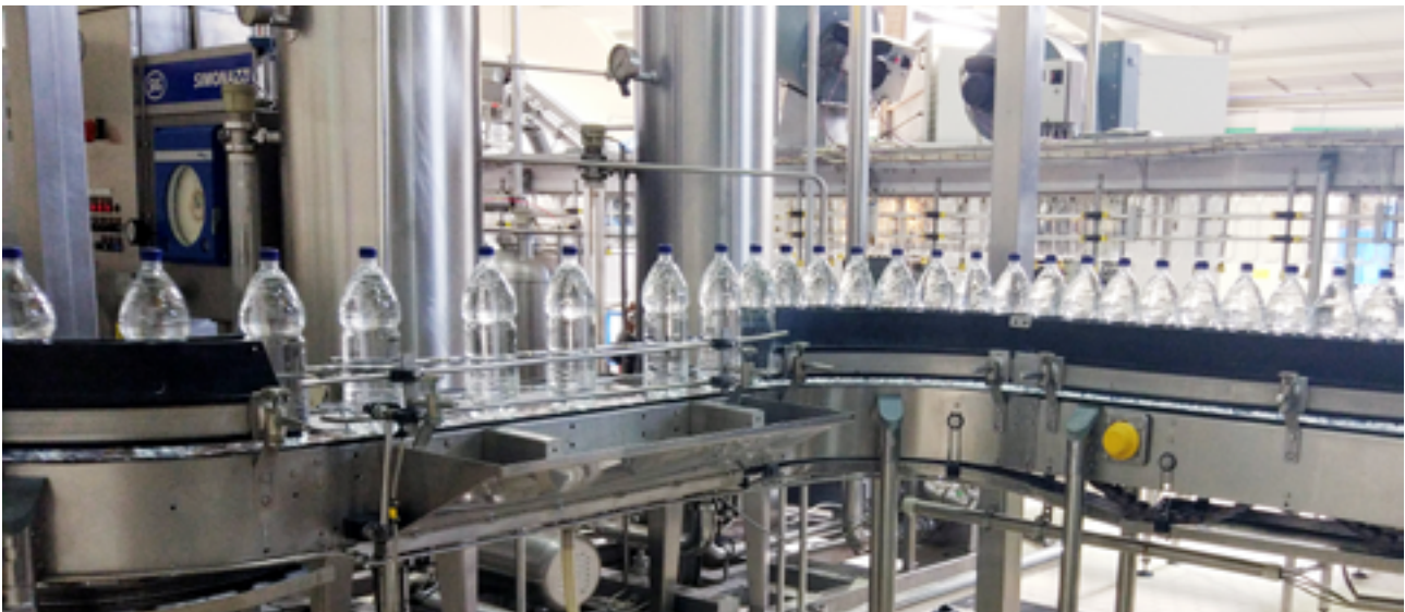
The new 2 L bottle line in operation, ozonated with Ozonetech's system to ensure sanitized bottles and highest quality water.
