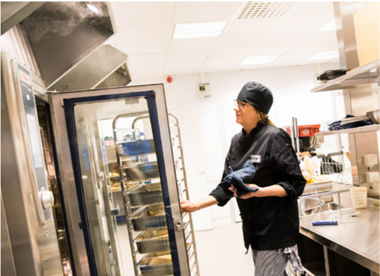
The ozone meets the greasy extract air right at the kitchen hood and treats it immediately.
