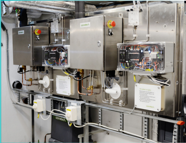
Ozonotech RENA 80 ozone system installation.
