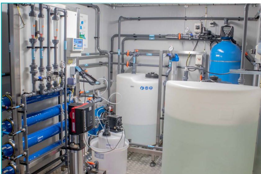
Water Maid N-series in operation.
