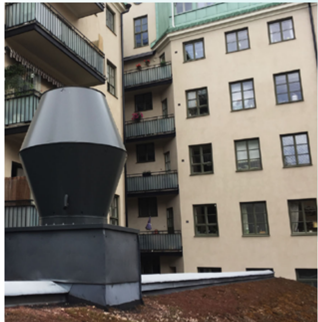
The point of discharge of exhaust air is close to a courtyard and the residents' balconies.
