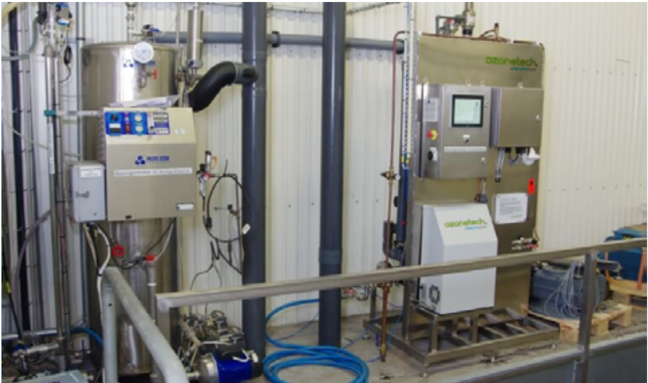
The Ozonetech RENA Vivo high-performance ozone system reduced the operating costs by 80%.
