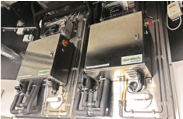
The fully automated wall-mounted RENA Kitchen Solutions with remote monitoring.
