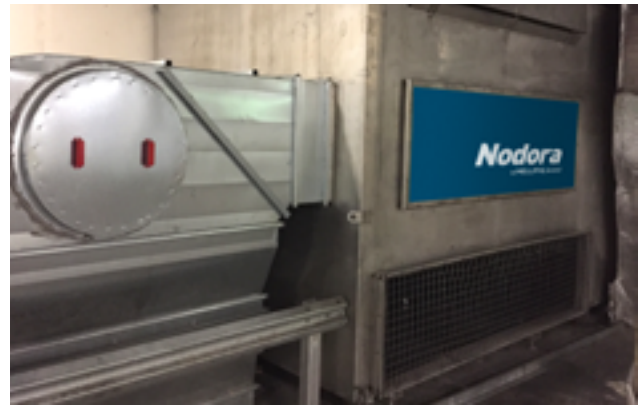
High-efficient odor removal system with multiple discharge points designed from scratch by engineers at Mellifiq.
