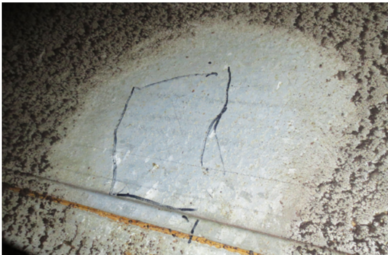
No grease accumulated on the cleaned test area after 12 months. Test and photo by Stena Line.
