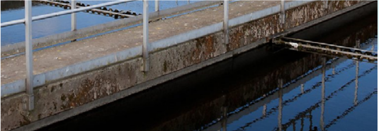
Sewage treatment plant in Tierp, Sweden.
